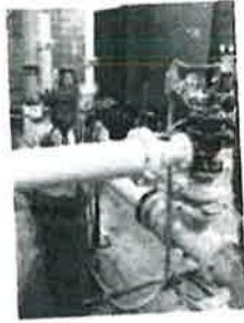
Plant Piping (Bypass)
