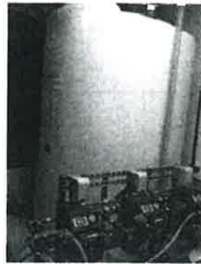
Chlorination Chem Pumps
